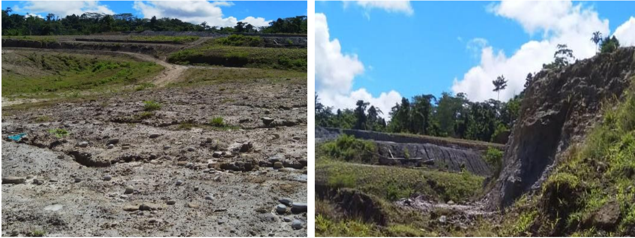
Figure 5 The planned upstream watershed for the built-up area has been partially leveled (left). Some of the lands is still steep and made like a ladder (right)
